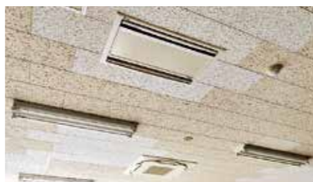
Ventilation units in the Kasuga Area lecture rooms
